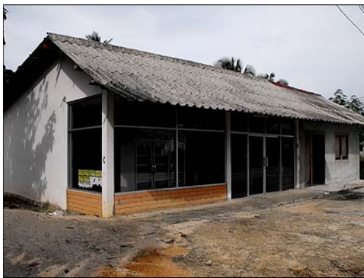
The old shop building we will have to renovate to make secure and usable as office/school room.
