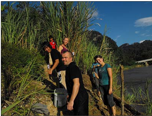
Some of the visitors helped gather rocks from the river for use in the concreting.
